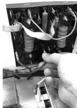
Disconnect at Diode Blocks
