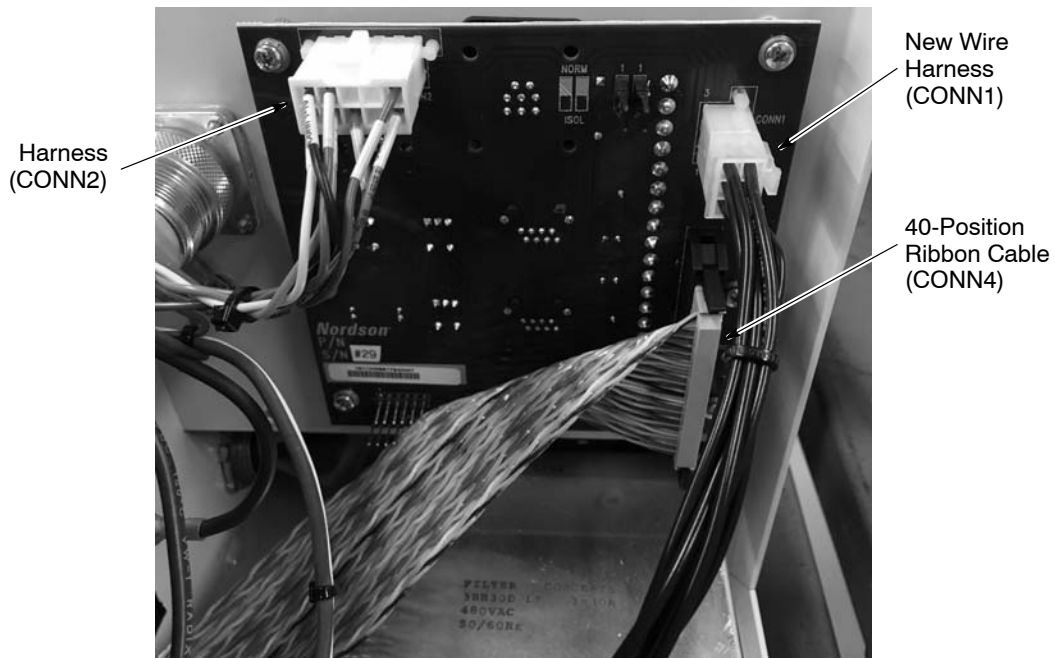
Figure 8 Installing New I/O Board
