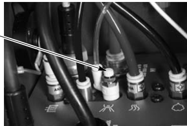
Figure 3-3 Electrode Air Wash Valve Location
