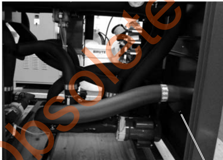
Process Water Strainer
